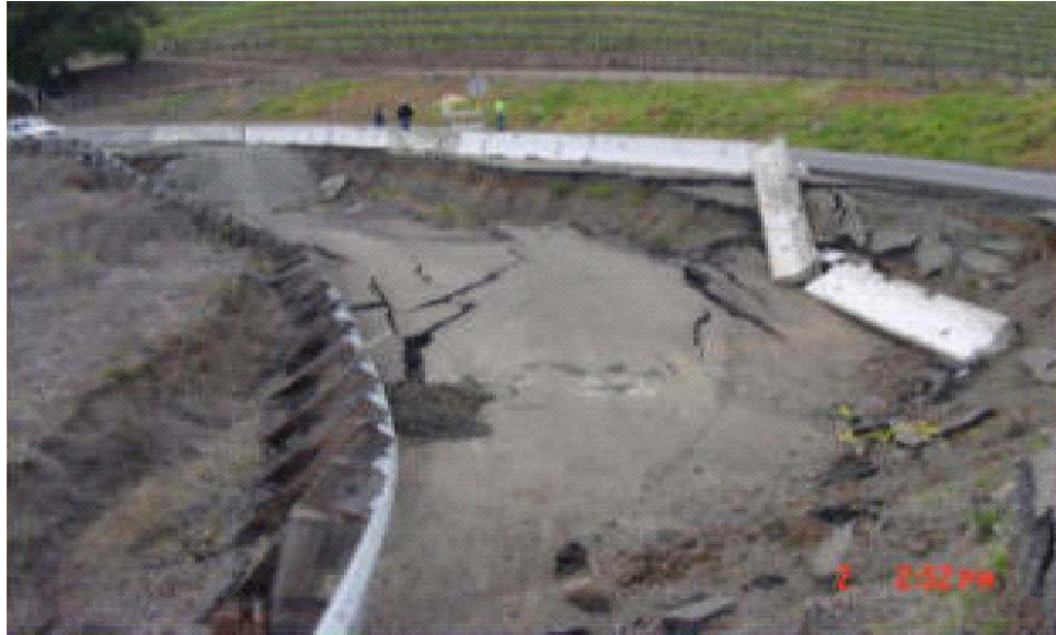
FIGURE 5. Landslide Damaged Section of Marina Drive, Ukiah, CA (12)
