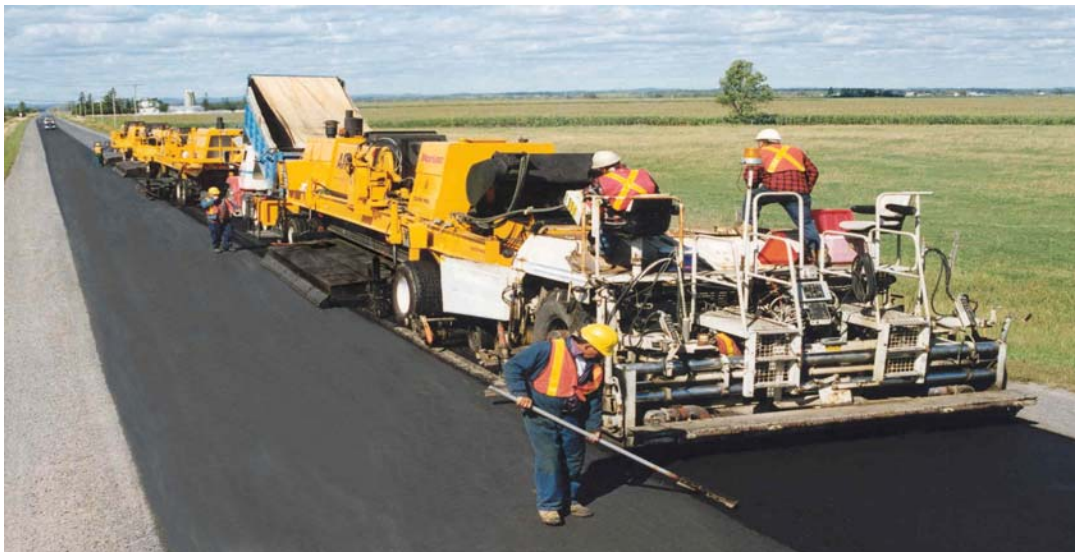
Figure 7 The current Martec AR 2000 Hot Air HIR Train After Re-Laying the Recycled Pavement
