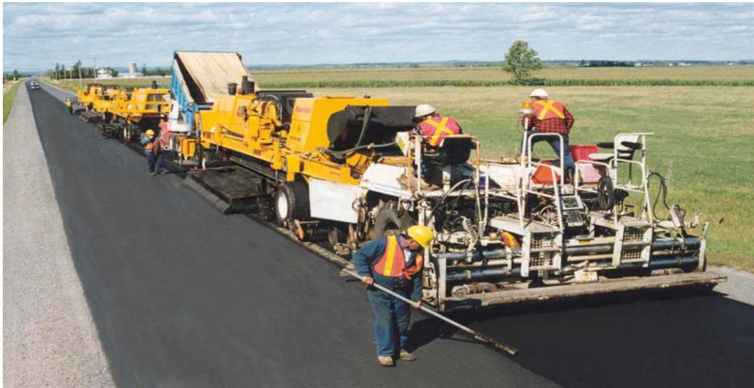
The current Martec AR 2000 Hot Air HIR Train After Re-Laying the Recycled Pavement
