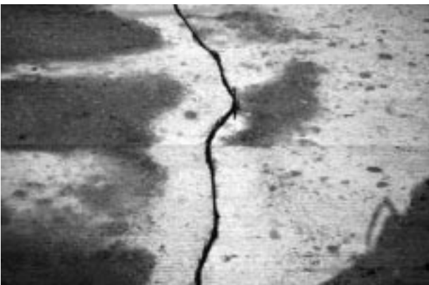
Figure 7.1. A freshly sawed crack.
