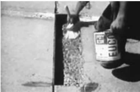
Figure 13.1. Application of bonding agent to the concrete surface – note the joint reforming medium.
