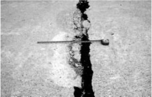
Figure 2.2. Moderate to severe spalling along a joint.
