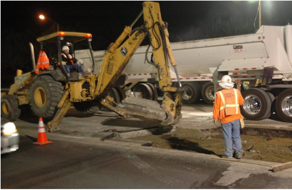
Figure 2. Damaged highway panel being removed.
