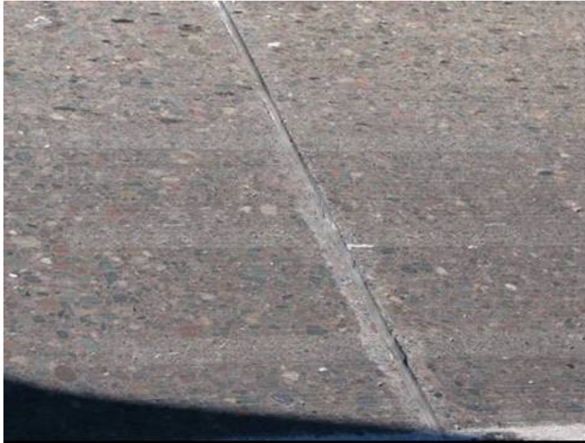
Photo 6. TH 23 slots with Mn/DOT 3U18 backfill mortar after 8 years.
