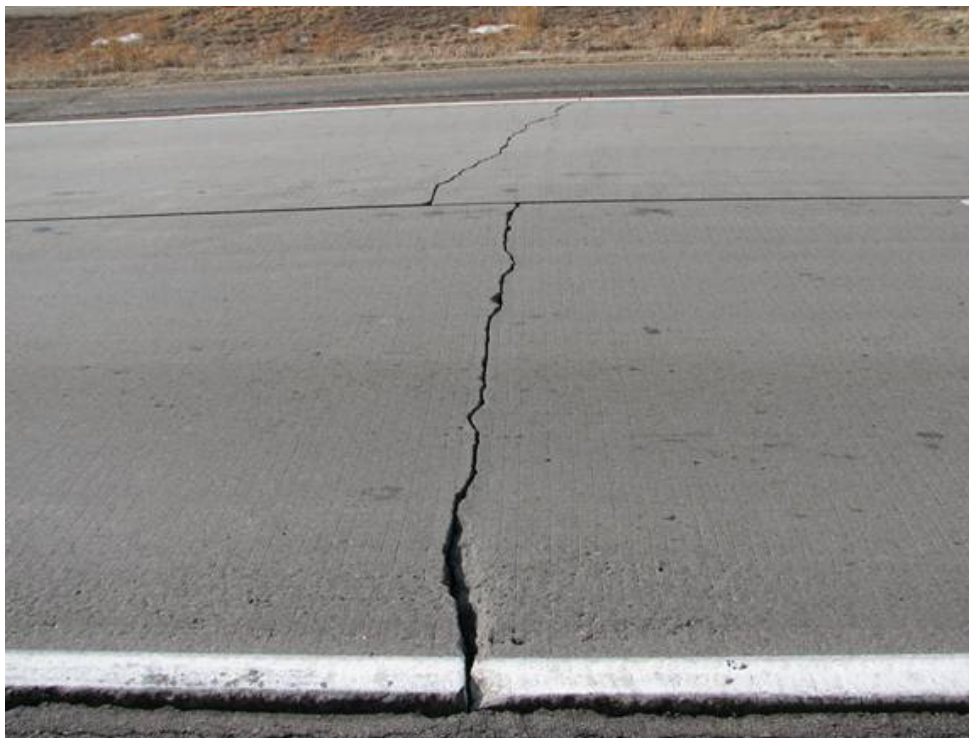
Photo 4. Faulted mid-panel cracks without retrofit dowels on TH 52.
