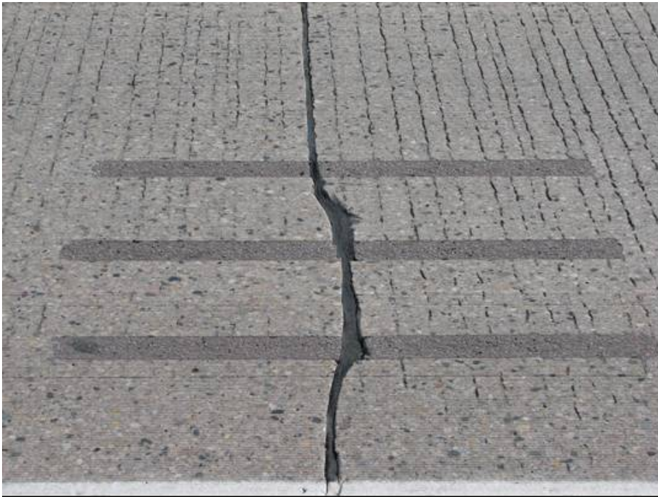
Photo 7. Typical condition of I-90 slots with PMQP backfill mortar after 7 years.
