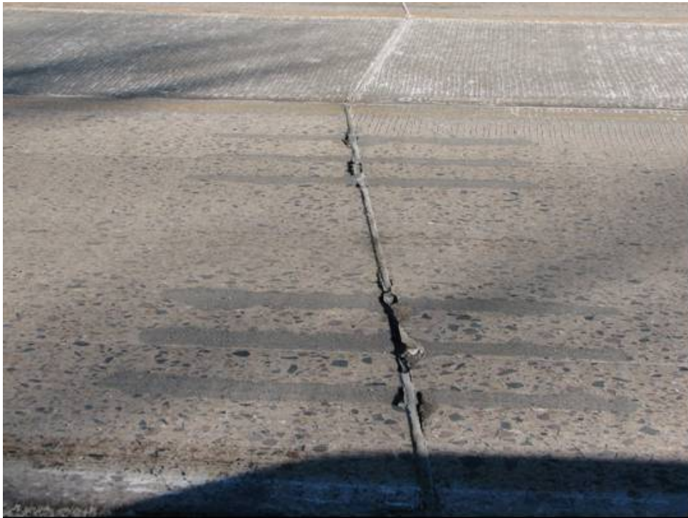
Photo 5. Backfill mortar distress near joints on TH 12.
