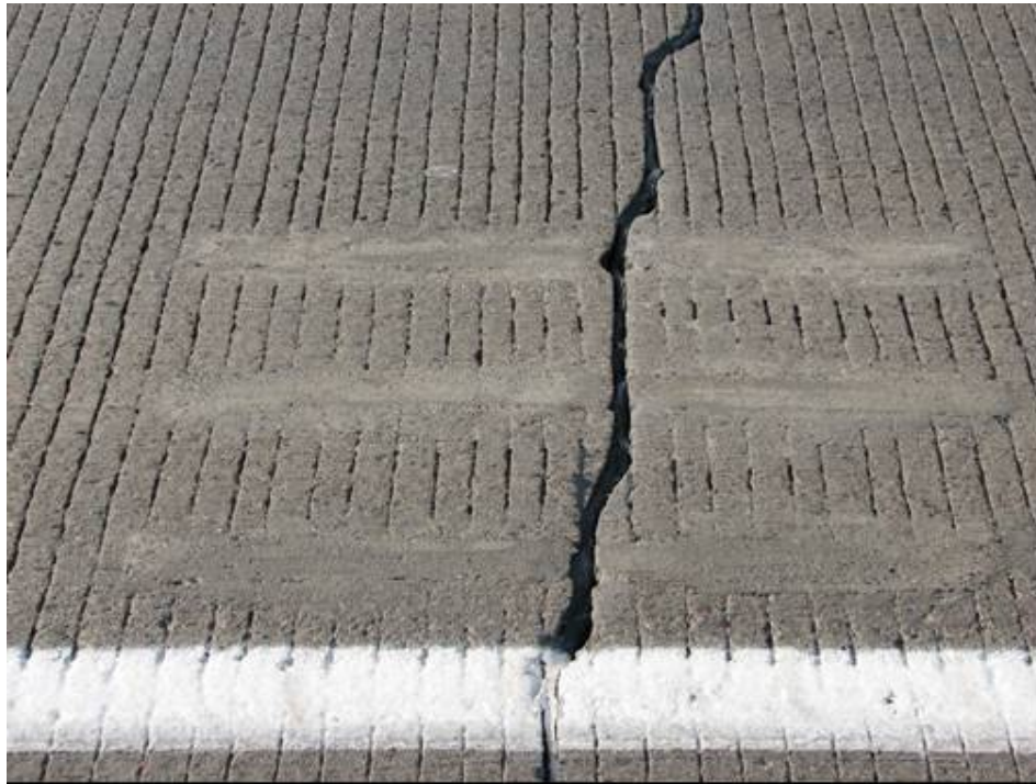
Photo 2. TH 52 slots with Mn/DOT 3U18 backfill mortar after 13 years.
