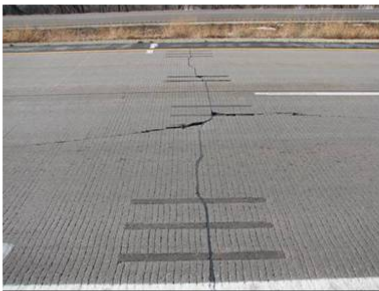
Photo 1. Distress in TH 52 retrofit dowel bars caused by longitudinal panel cracks.
