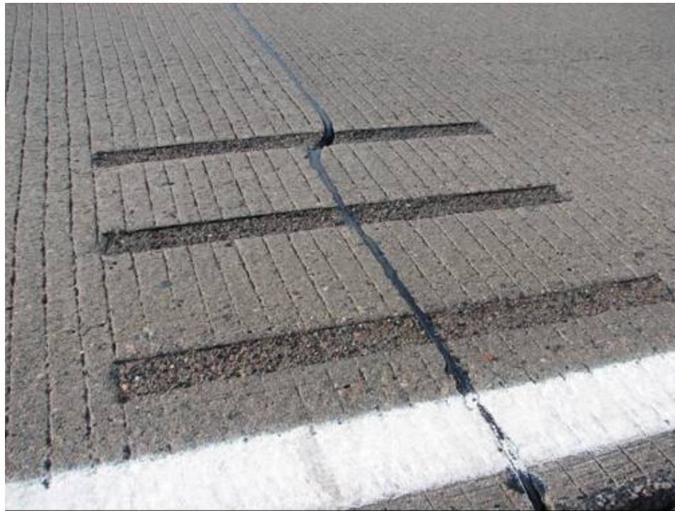
Photo 3. Loss of PMQP mortar near surface of slots on TH 52.
