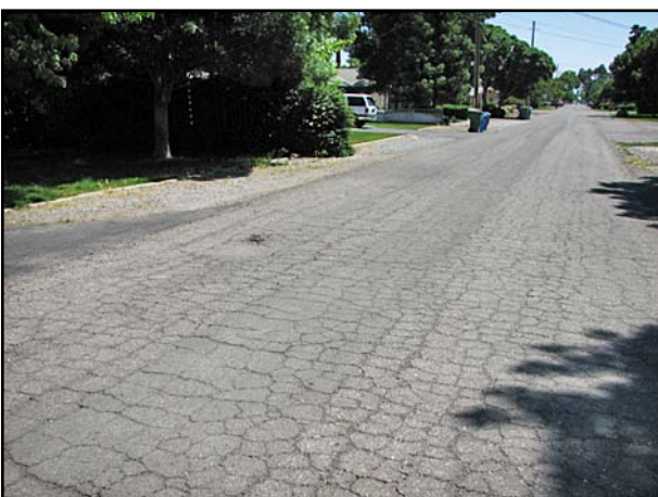
Severely alligator cracked pavement in the community of Sutter. This location received a PME 3/-8" chip with micro-surfacing
