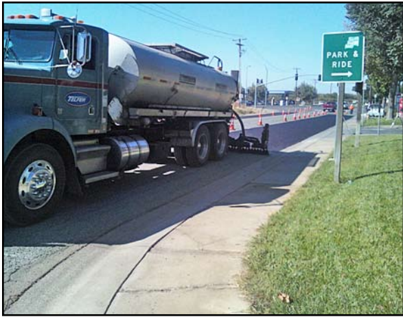
Placement of a flush coat on Bogue Road. The flush coat actually increased rock fly, so flush coat work was eliminated from subsequent locations
