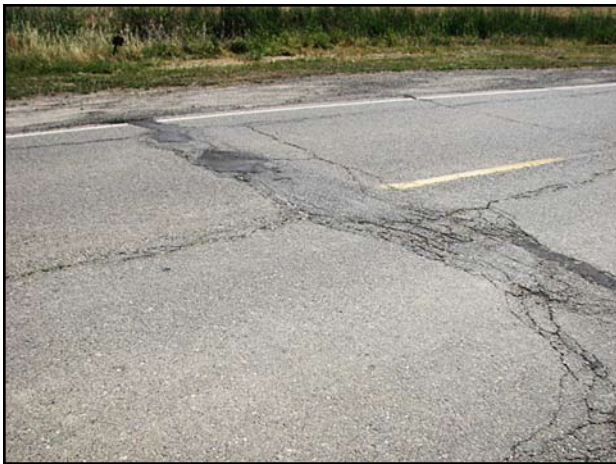
Severe transverse block cracking on Central Street in the community of Meridian. In the future, the County intends to do more AC pavement repair and crack sealing prior to placing seal coats over locations like this
