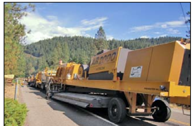
Third Generation hot in place recycling train in Big Bar area of California
