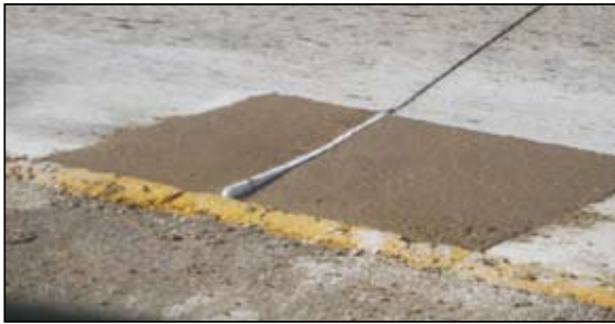
Larger patch area, I-10 east-bound lanes.
