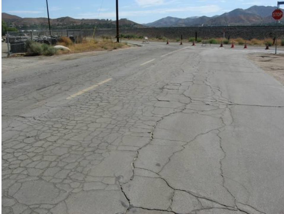
Figure 3 High severity alligator cracking on Smith Avenue before Soledad Canyon Road
