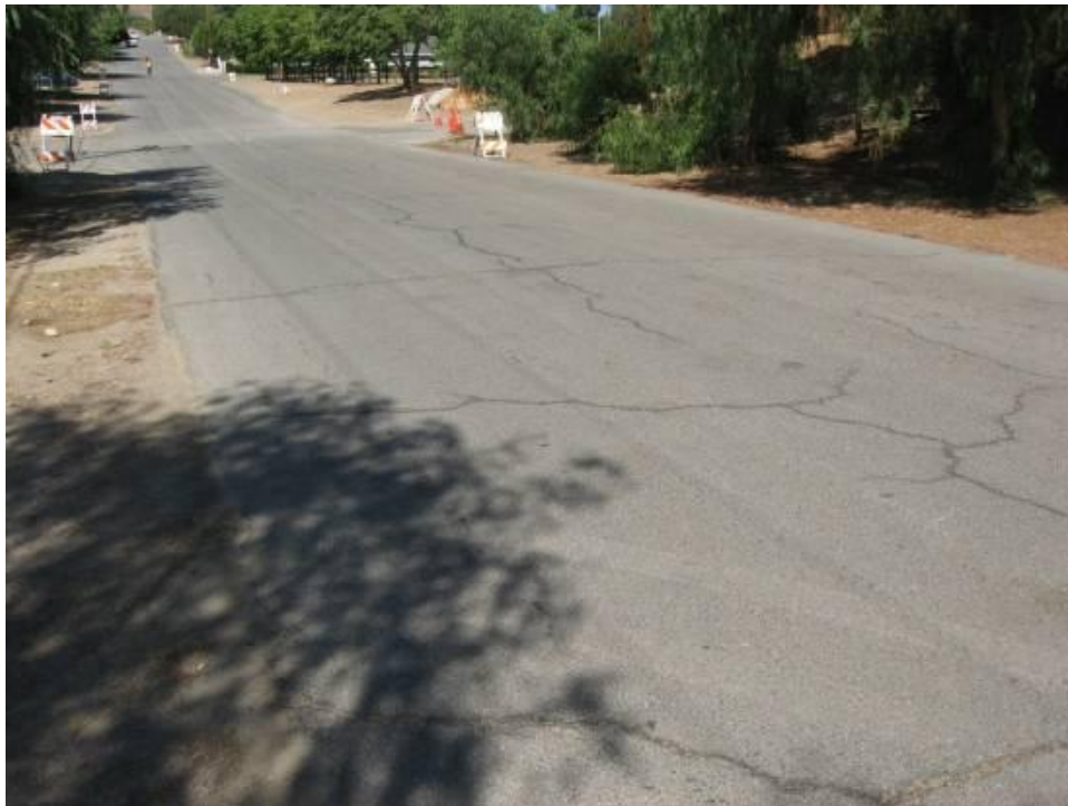
Figure 2 Longitudinal and transverse cracking on Smith Avenue
