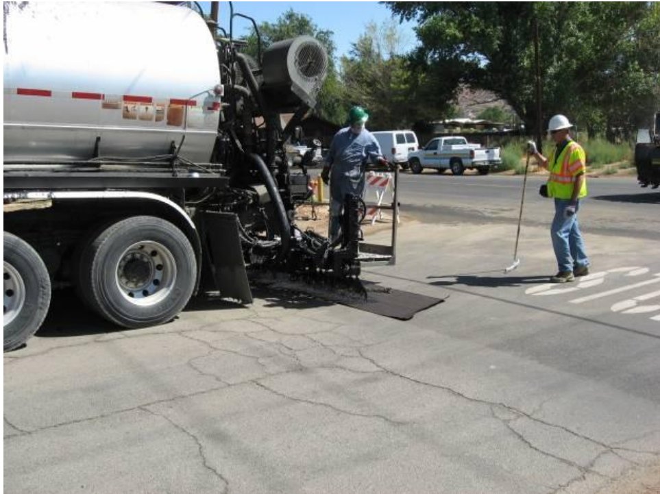
Figure 5 Tarp being used under the spray bar at the beginning of a new section
