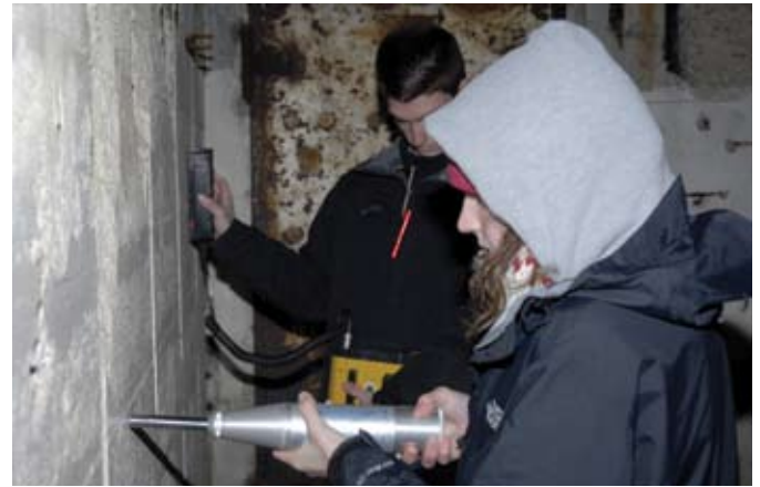
Fig. 4: Inside the observation post, Courtney Sheehan tests relative concrete strength with a Schmidt (rebound) hammer while Chad Golden uses a cover meter to determine location, size, and cover of embedded reinforcing
