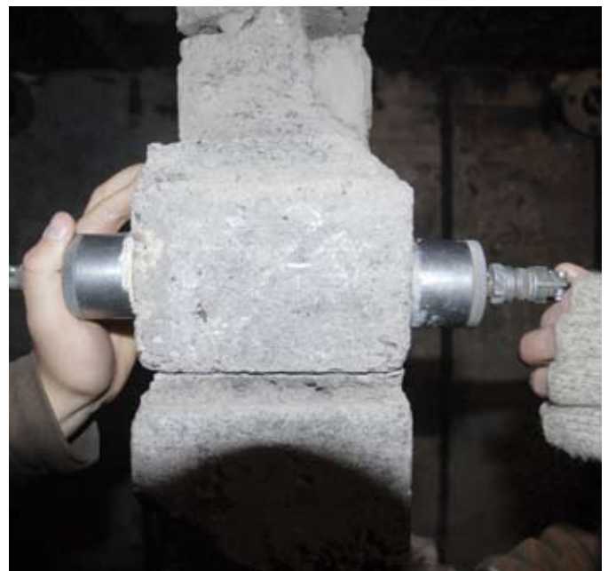
Fig. 8: Close-up of ultrasonic pulse velocity test on an observation post interior wall with two-sided access
