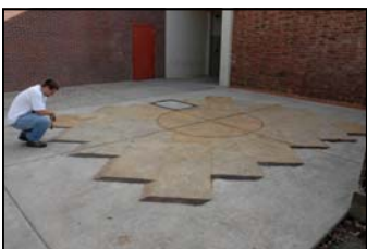
Integrally colored slab poured, textured, 3D stained, & sealed by Chico State CIM Decorative class, Chico State campus, Oct. 2008.
